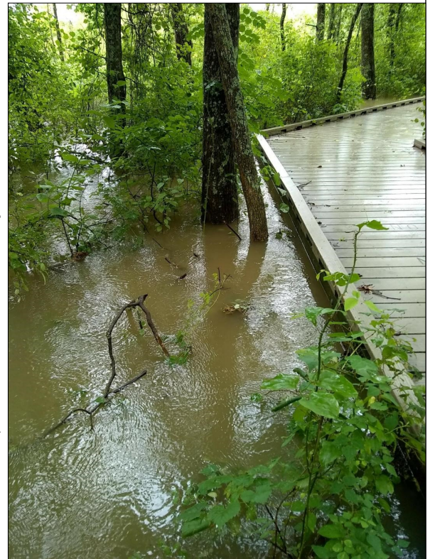
Water level at the beginning of the boardwalk after the July 8, 2019 rain event.
